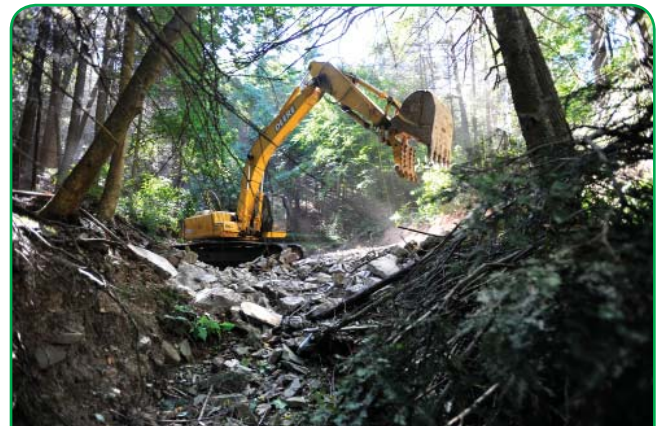
Contractors from Aquatic Resource Restoration Company removing rubble from the Musser Gap site on day two of the dam removal and restoration project.
